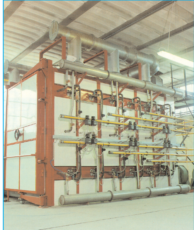
Sanitary fittings baking furnace with "Nozzle Mix" burners (Intercer)
