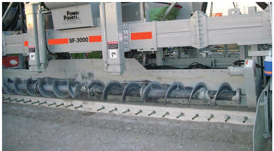
The sideforms widen allowing the machine to begin paving off an existing header. Hand tie-in work is minimized resulting in a better quality and smoother pavement.
