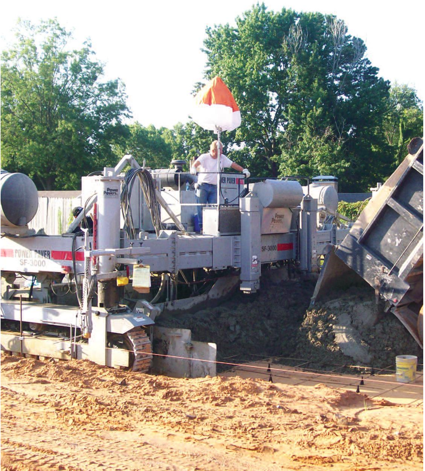
SF-3000 has the size and power to handle large volumes of concrete. Here it is paving over steel reinforcement.
