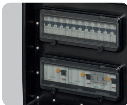
Single-pole MCB for three-phase current outlets
