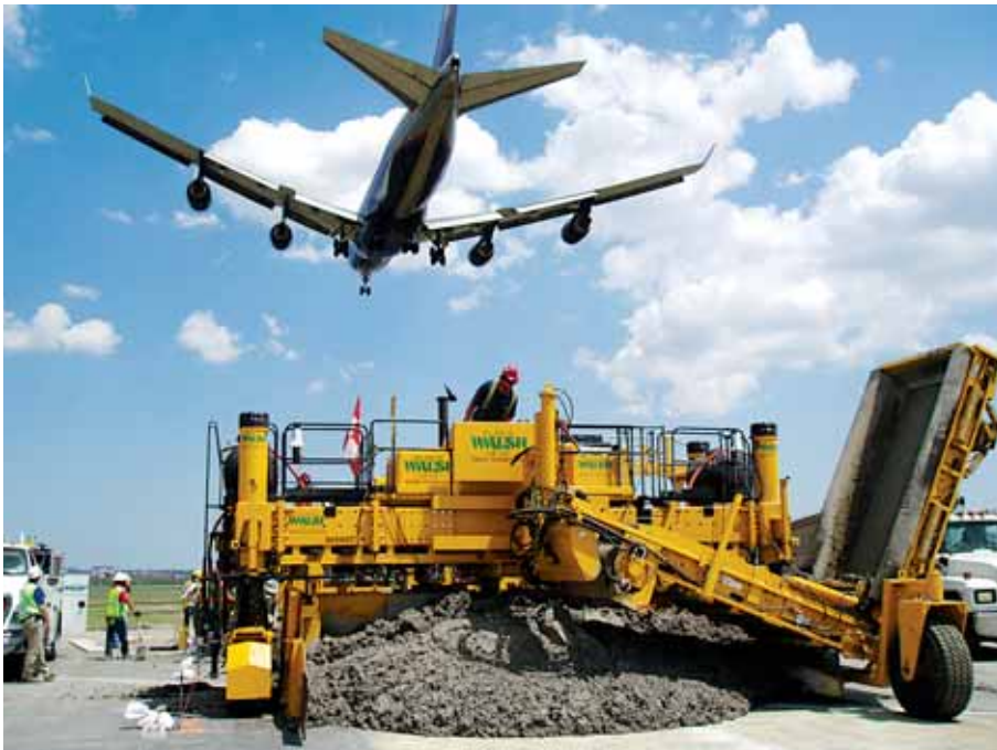
The GOMACO PS-2600 places concrete on one runway section of the airport, while other runways can remain open for planes to take off and land.
