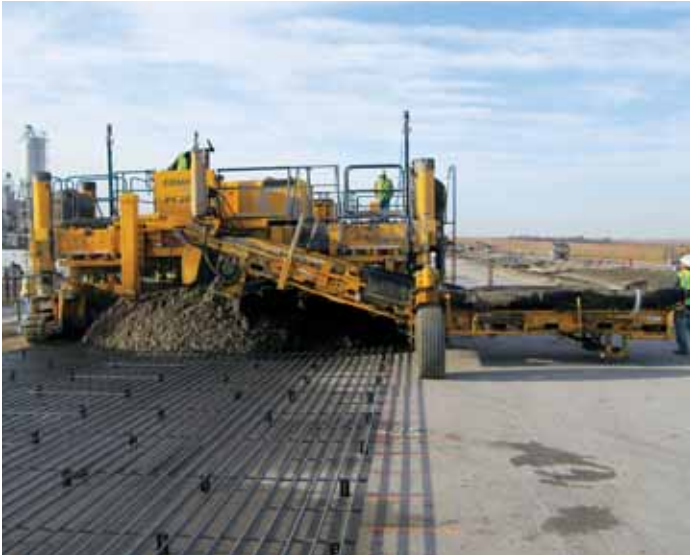
The GOMACO PS-2600 paver/spreader places concrete over continuous steel reinforcing on a toll road in Texas.
