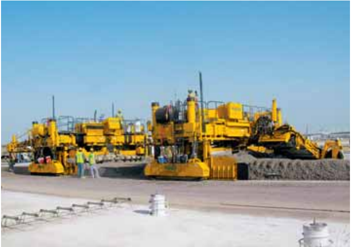
The GOMACO PS-2600 and GHP-2800 make up the paving train on this airport. This runway is being paved 25 feet (7.62 m) wide.
