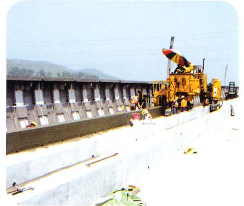
Anti-Derailment Barrier in Hong Kong.
