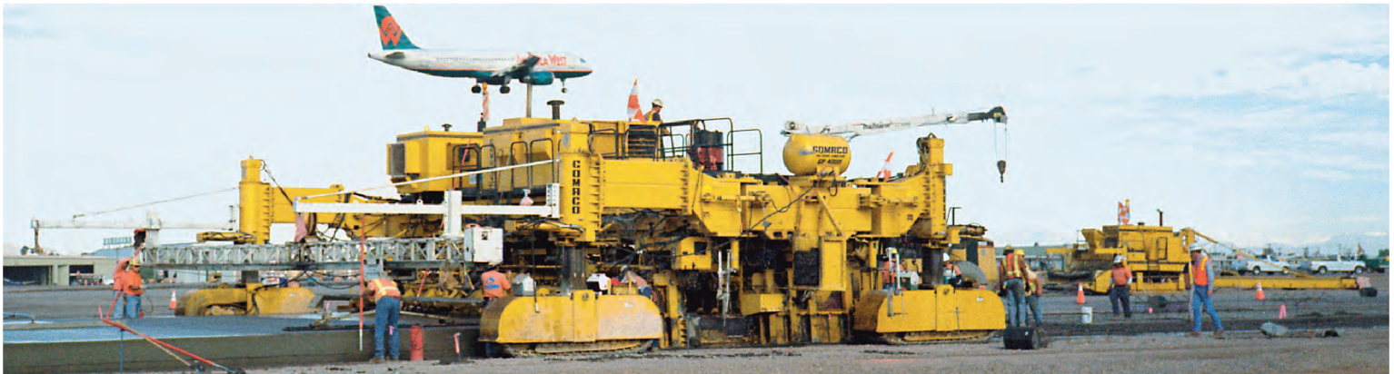
This GP-4000 four-track slipform paver, equipped with the GOMACO patented In-The-Pan Dowel Bar Inserter (IDBI) system, meets all specification requirements on the Sky Harbor Airport in Phoenix, Arizona. High production on runways and aprons is achieved while slipforming paving depths up to 19 in. (483 mm) and 50 ft. (15.24 m) wide.
