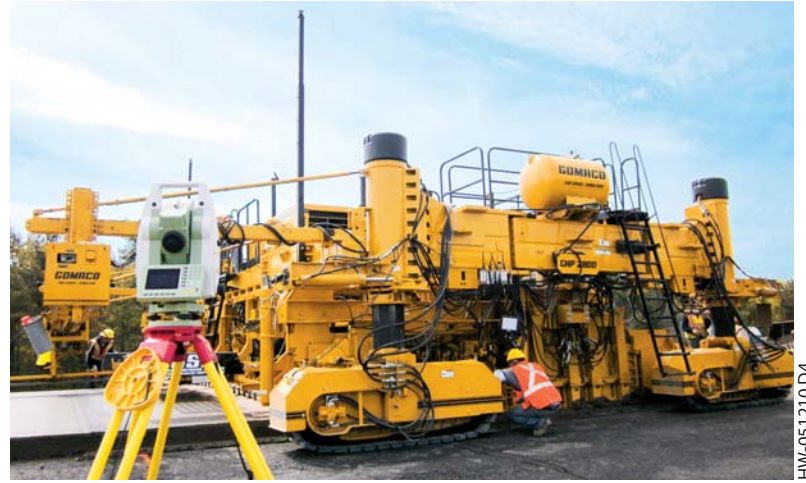
The paver is equipped with Leica Geosystems 3D, two paver-mounted GSI units, and an IDBI for placing the dowel bars for the transverse joints.
