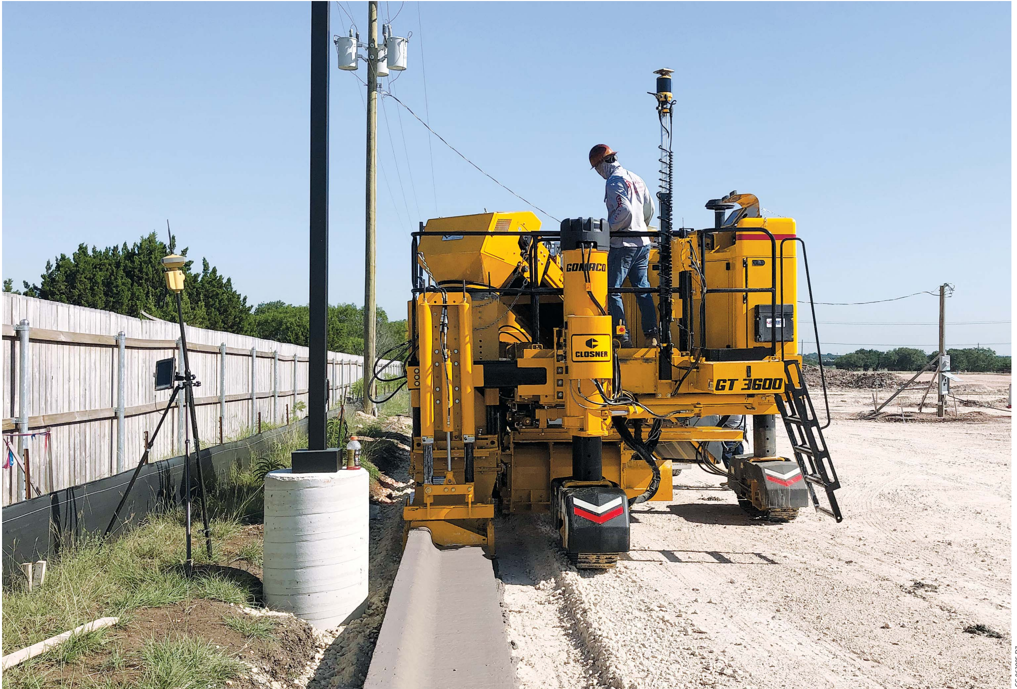
3D machine guidance helps achieve minimum clearance eliminating the need to set stringline on projects where existing utilities create challenges.
