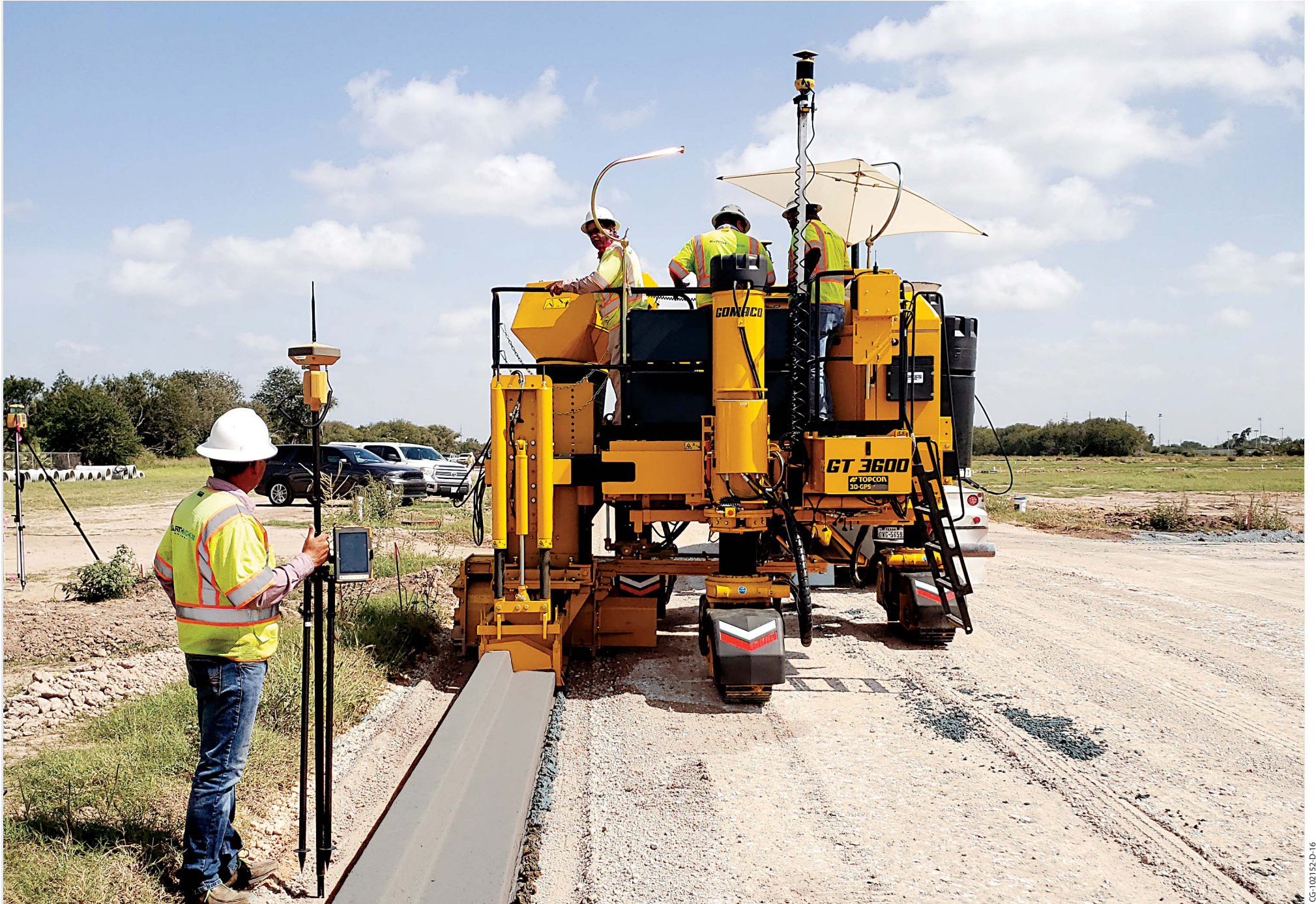
An 18 inch (457 mm) curb and gutter is slipformed using 3D machine guidance by the Xtreme GT-3600 in a new residential development.
