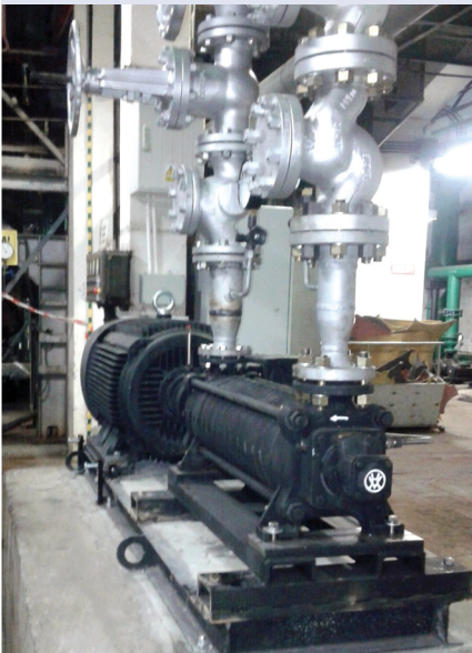
Heat and power generating plant in Mielec - WH pump
