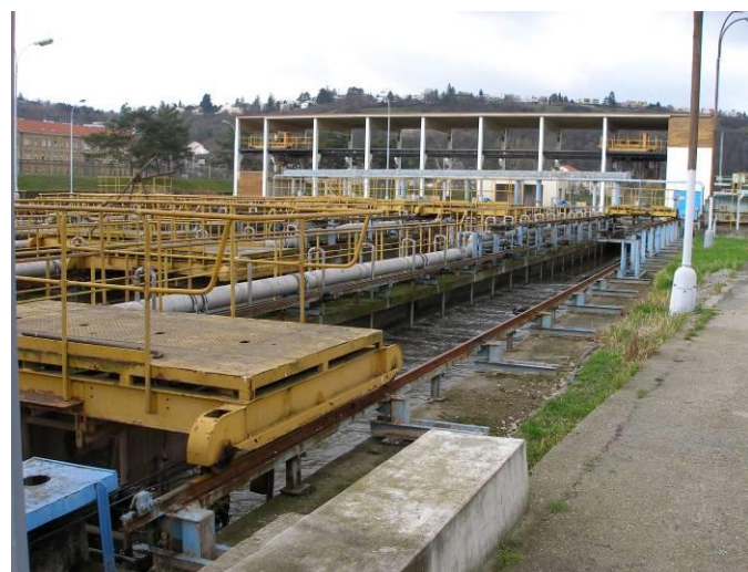
Water treatment plant - sand traps
