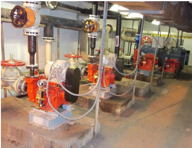
2 x MAPE 50, 3 x Mape 100, Transportation of water with sludge. Installation of the Automatic seal protection ASP 21
