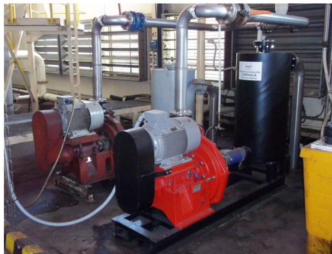
2 x MAPE 100, Transportation of water with fiberglass remains. Installation of countershaft tank
