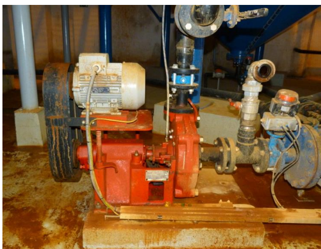
MAPE 50, Mine water treatment plant – transportation of mine water with sludge
