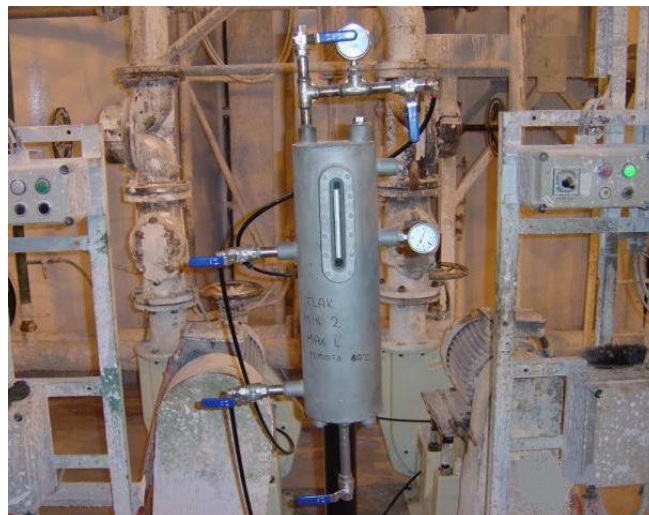
2x MAPE 100, Transportation of whitewash Installation of thermosiphon on the closed circuit of running water of two fold mechanical seals
