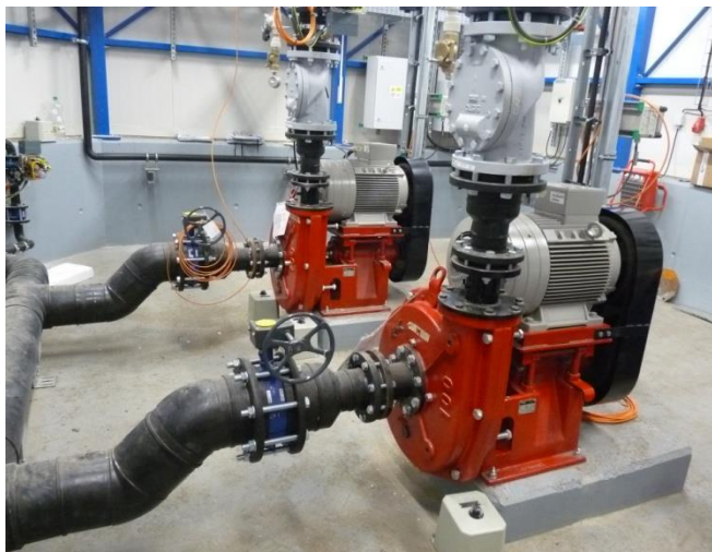
2 x MAPE 100, Power plant - transportation of processed water
