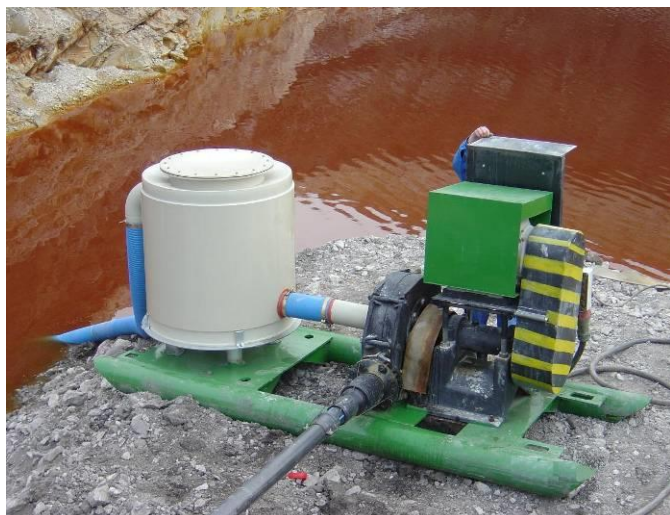
MAPE 150, Transportation of mine water during the extraction of ceramic substance. Installation of countershaft tank
