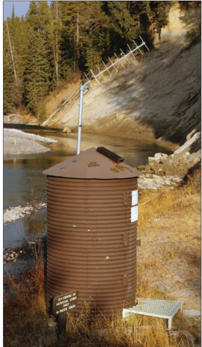
The TX320 transmitter offers reliable GOES communications for remote gaging stations.
