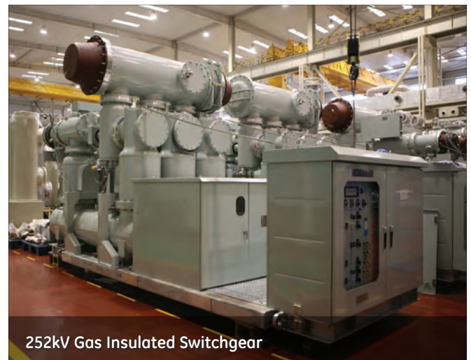
252kV Gas Insulated Switchgear
