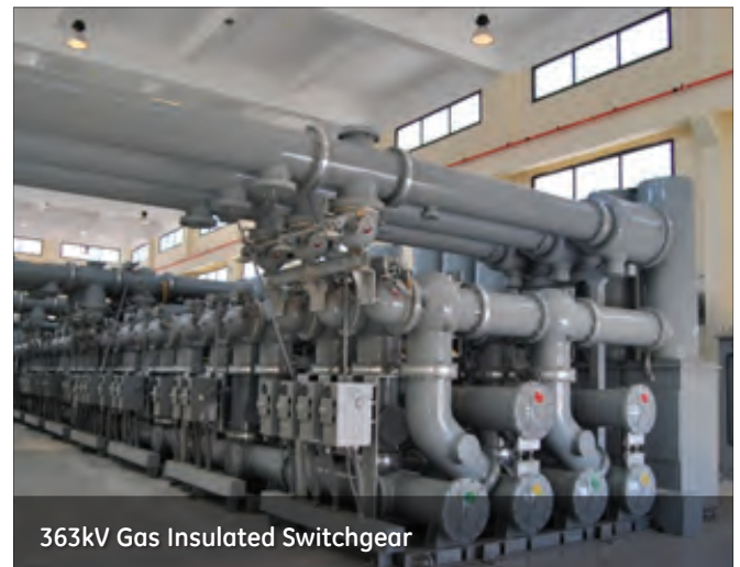
363kV Gas Insulated Switchgear at Golmud Substation
