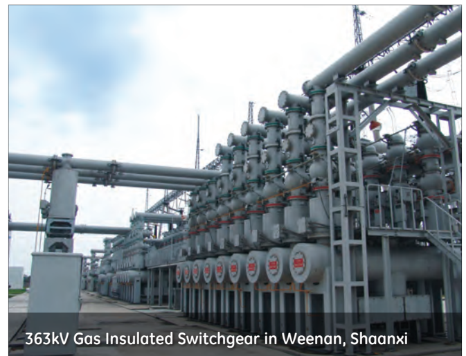
363kV Gas Insulated Switchgear
