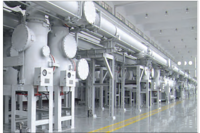
550kV Gas Insulated Switchgear
