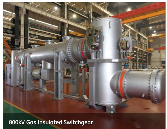
800kV Gas Insulated Switchgear at Lan Zhou Substation
