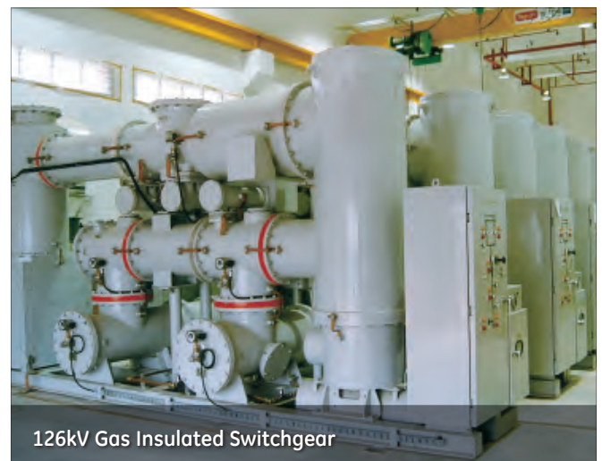
126kV Gas Insulated Switchgear
