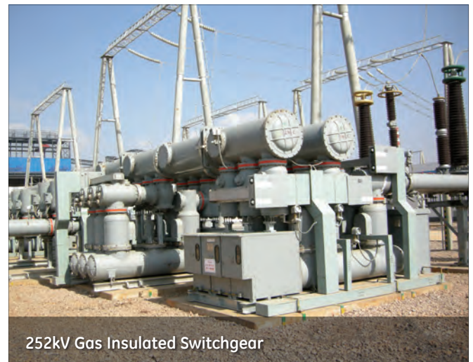
252kV Gas Insulated Switchgear
